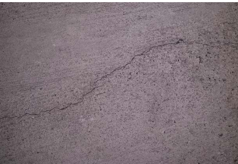
Plastic shrinkage cracking
